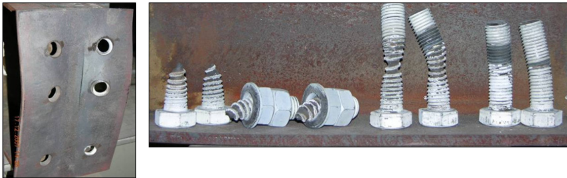
Figure 7: Failure of end-plate connection at 550°C / 650°C.
