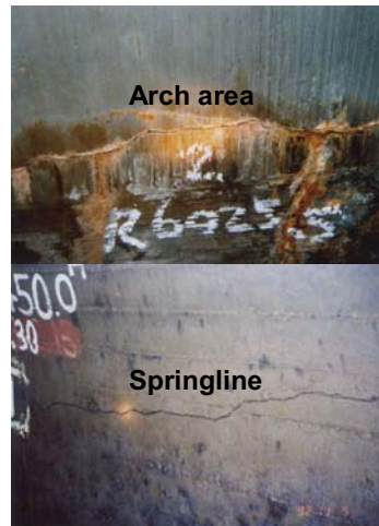
Photo 1 Longitudinal cracks observed in an aging waterway tunnel
