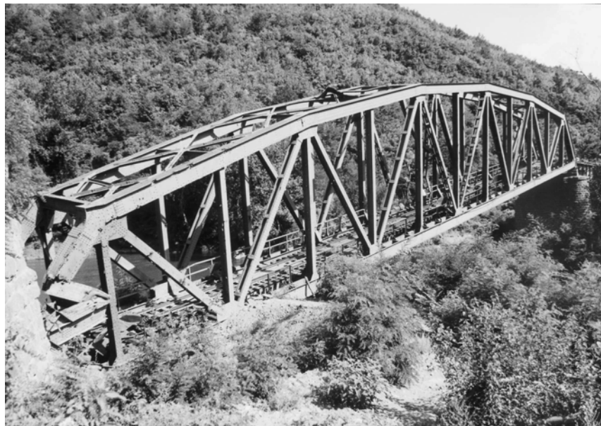
Figure 2: Destroyed bridge Pivnica
