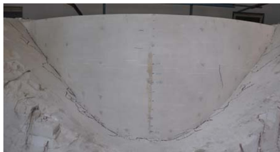
Figure 7. The final crack status of upstream dam surface
