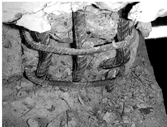
Figure 1: Column base damage of concrete and reinforcing bars in low cycle fatigue test on reinforced concrete column prototype [6].
